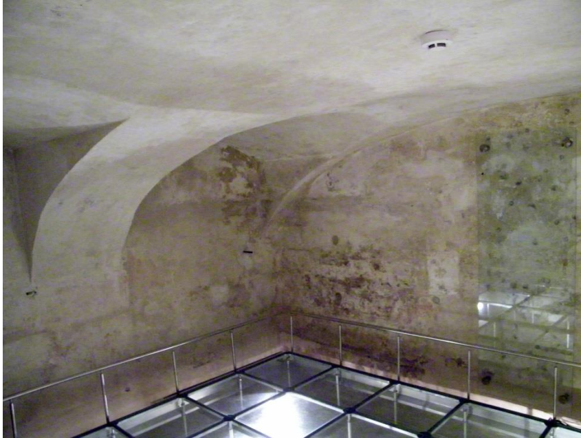
The KGB prison's execution chamber. Plexiglas on the wall to the right covers several bullet holes in the concrete wall.
