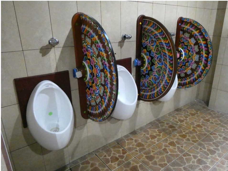
The facility features these very decorative, hand-painted urinal separators, which gave me a new picture for my collection of foreign bathroom photos.
