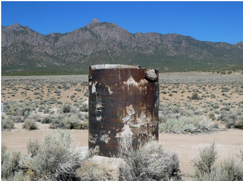
The top of the steel tube, sealed with concrete. You can see how much the earth dropped here.
